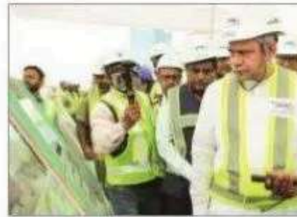
Minister of railways Ashwini Vaishnaw visits the construction site of Bandra Kurla Complex Station
